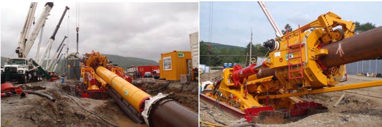
Figure 3. Installation of a 42-inch steel pipe in New York, August 2011. On the left, the pipe thruster is pushing the MTBM forward while the trailing steel pipeline can be seen supported by cranes. On the right is a close-up view of the pipe thruster in action. Photos provided by Herrenknecht AG.
