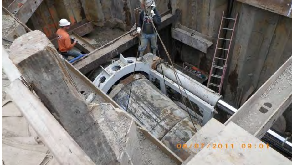
Figure 10. TBM Pulled into the Shaft with an 800-ton jacking frame operating in reverse
