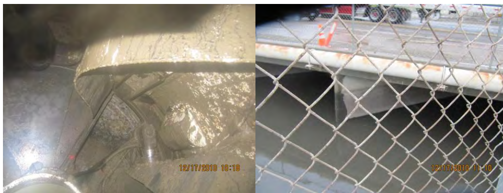
Figure 8. Concrete Obstruction beneath the OID and a view of the wall supporting the roadway above the drain
